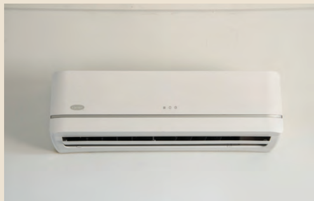
Ductless air source heat pump indoor unit.
