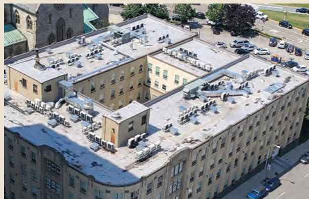
Commercial air source mini-split heat pumps at the Police Apartments in Buffalo, NY.
