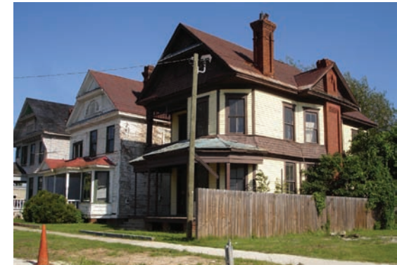
Some urban housing stock has fallen into disrepair
