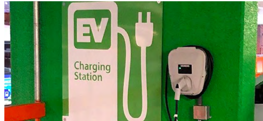
In January 2019, Anchorage Community Development Authority installed an electric vehicle charging station in an EasyPark garage in downtown Anchorage. The charging station will be free to use through the end of 2019. 31 Photo credit: Easy Park
