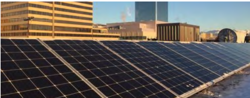
25-kW solar installation on a commercial building in downtown Anchorage. Photo credit: Arctic Solar Ventures
