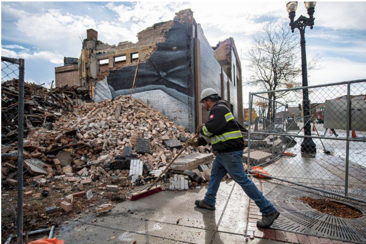
Figure: Demolition of blighted building on Broadway St. in Gary, IN on November 5, 2020. Source: https://www.chicagotribune.com/suburbs/post-tribune/ct-ptb-gary-downtown-demolition-st-1107-20201106-fsap77u64zfzhkdfmhmbq2ypry-story.html
