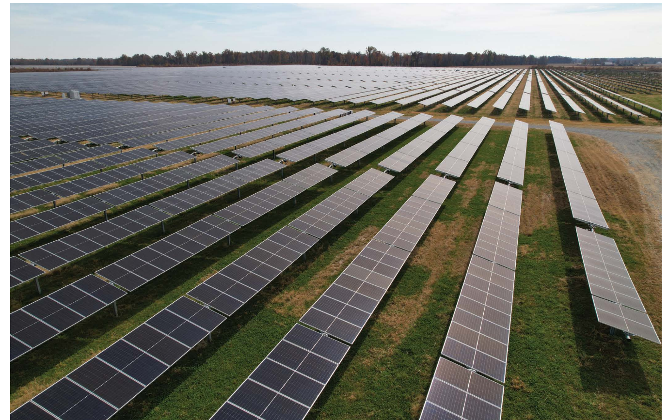
The New Market Solar Array provides electricity for City operations and the residential aggregation program. Photo courtesy of Algonquin Power & Utilities Corp.
