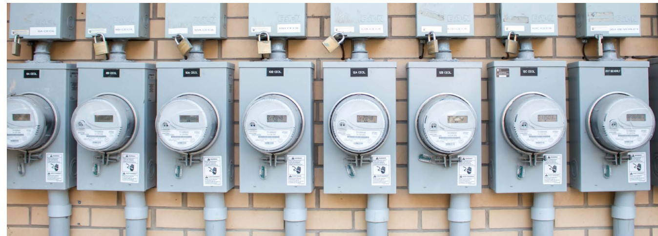
Electric meters on a multi-family building.
