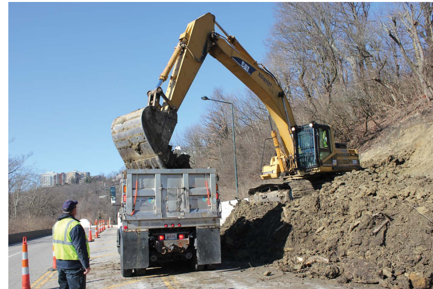
Cleanup of a landslide onto Columbia Parkway. Photo courtesy of City Staff.
