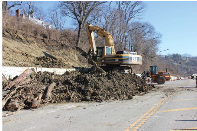
Landslide into Columbia Parkway in 2016. Photo courtesy of City of Cincinnati.
