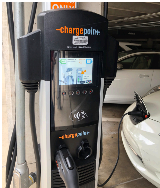
Electric Vehicle charging station at the Charlotte-Mecklenburg Government Center parking deck
