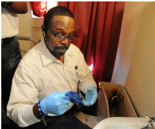
The Birmingham Water Works Board repaired leaks for over 200 customers during its Fix a Leak Week program. (Photo: Linda Stelter, Birmingham News.)
